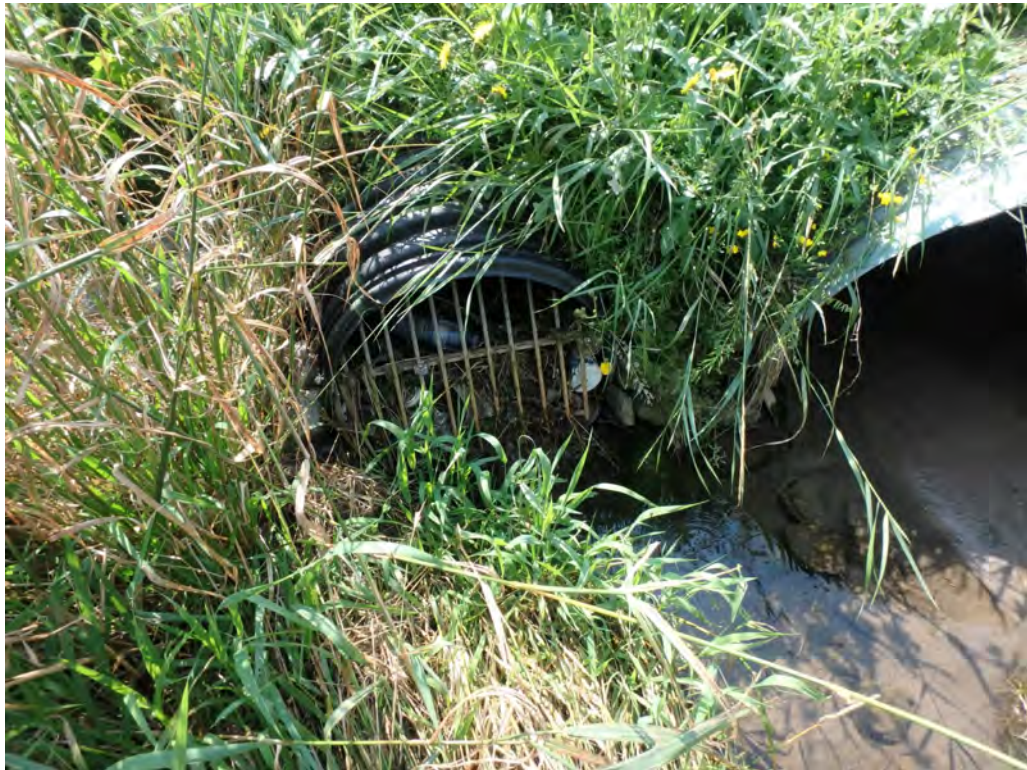
Photo 16: Habitat Zone 3, photo showing CSP, and plastic culvert blocked with debris and litter. Photo facing upstream (south) (Photo Date: July 22, 2021)
